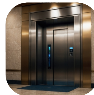
Lift : Kone / Johnson
